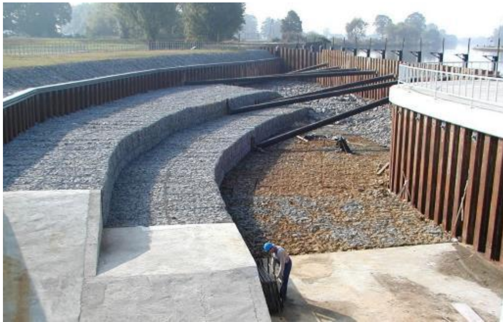
Figure 7: Shaping the inlet canal of Januszkowice SHP (1.5 MW) - Oder river, Poland (source: IMP PAN archives)
