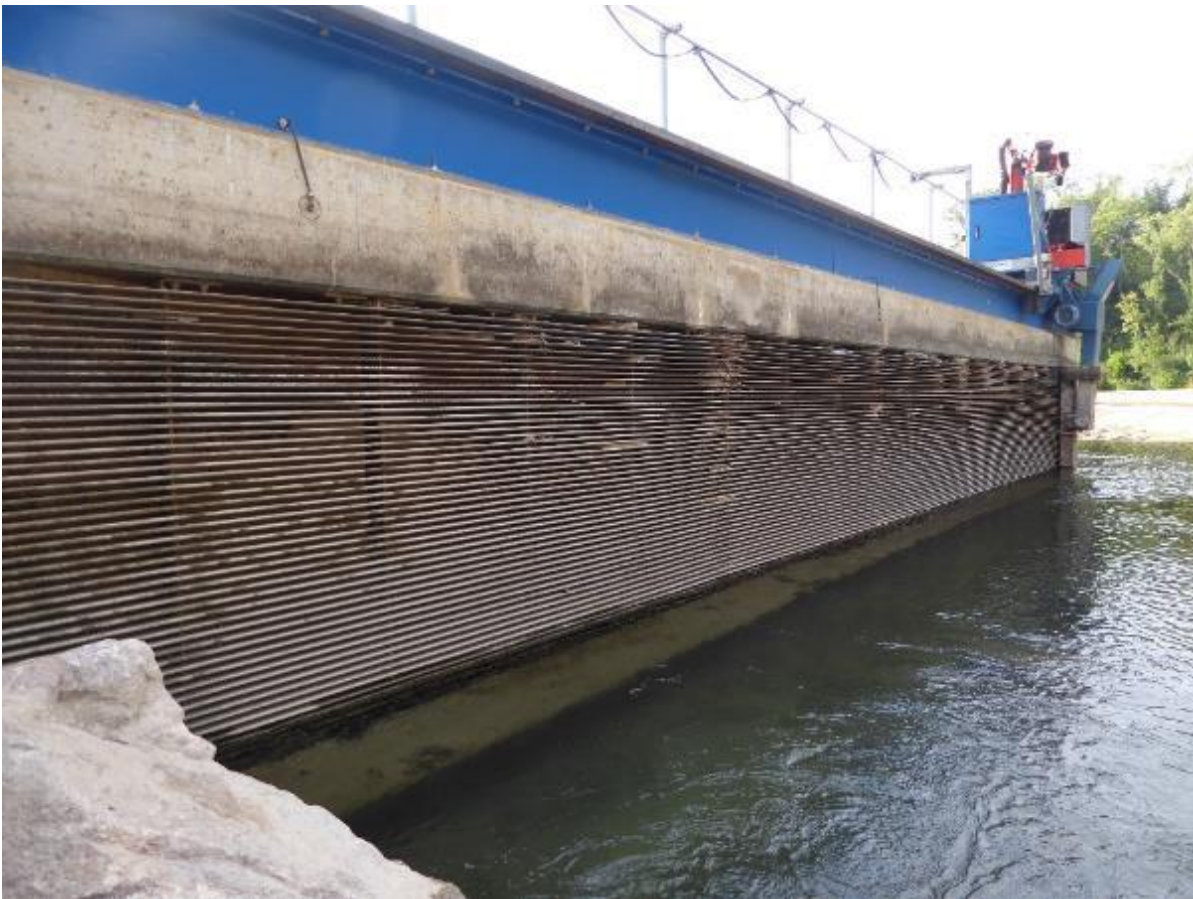
Figure 88: The horizontal bar rack of residual flow HPP Schiffmühle, Switzerland, during reservoir drawdown in July 2018 (source: J. Meister, VAW)
