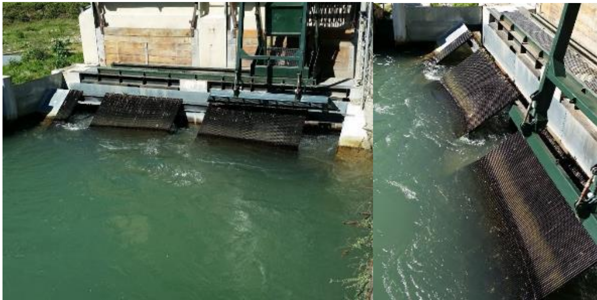
Figure 87: Inclined bar rack with openings to the bypass channel system (source: P. Rutschmann)
