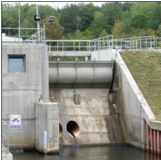
Figure 64: Weir crest hinged flap gate at Rzeczyca SHP - Wierzyca river, Poland (source: J. Steller)
