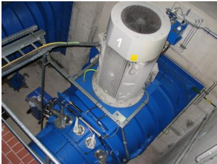
Figure 30: A typical compact unit with bevel speed increaser. Oborniki SHP, Poland (source: IMP PAN archives) Induction and permanent magnet generators are used among others in Hydromatrix and StreamDiver units delivered by Andritz Hydro (Figure 31) and Voith, respectively Cui et al. (2007), Keuneke (ed.) (2014) and Voith
