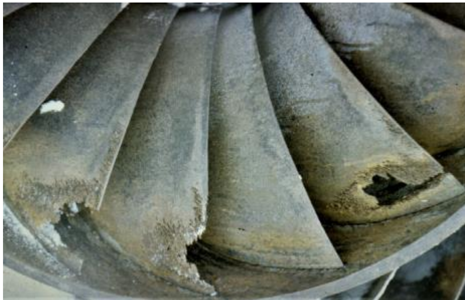
Figure 13: Extensive cavitation damage at the suction side of a small Francis turbine runner (1970s, source: IMP PAN archives)
