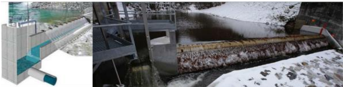
Figure 91: Coanda water intake illustration and example of Coanda water intake of Escouloubre (977 m altitude) on the Aude river, France (Source: AFB)
