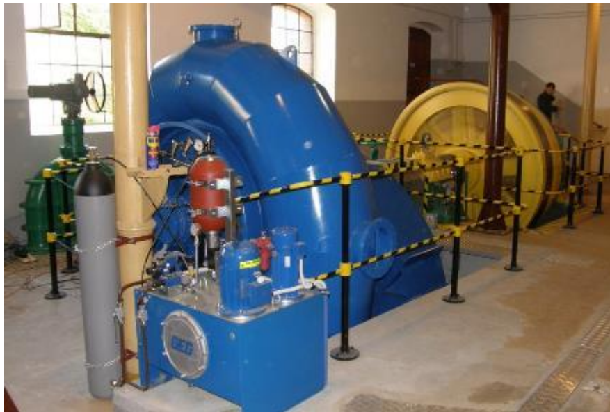
Figure 20: A modern Francis turbine in a refurbished Polish hydropower plant (source: IMP PAN archives)
